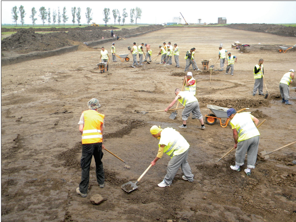
Fig. 37. Photo taken during the excavation conducted in the LBA settlement of Şagu-Site A1_1 (2010) (photo by the authors).
